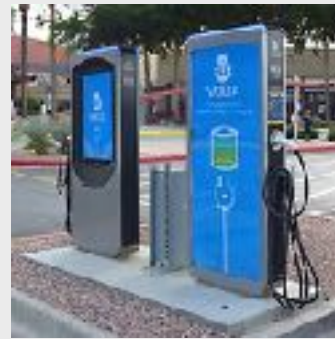
Electric Vehicle Infrastructure
