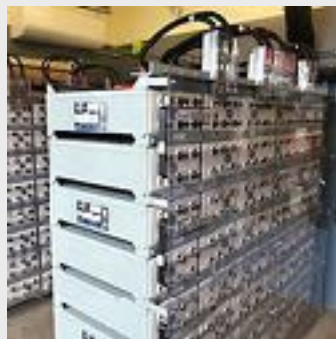
Backup Power & Storage
